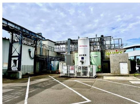
Wastewater treatment facilities (Head Office/Factory)
